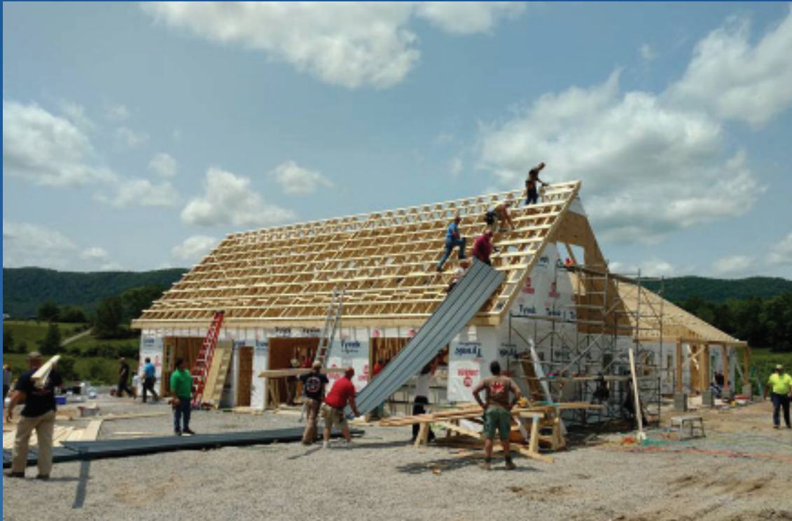
Volunteers from A Soldier's Journey Home (ASJH) start installation of roofing tin on the Wounded Marine House Build project for Lance Cpl. Cody Evans' new home May 2016. (Photo courtesy of ASJH Facebook page).
